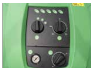
CONTROL PANEL WITH INDICATOR LAMPS
