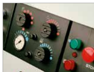
CONTROL PANEL PROVIDED WITH EMERGENCY SHUTDOWN
